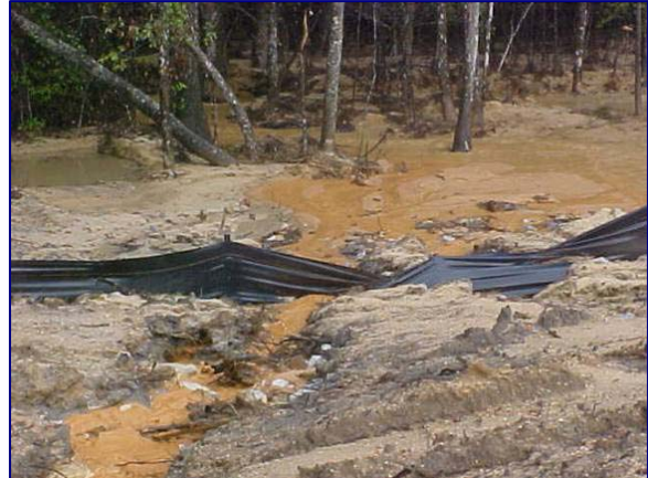
Failing sediment protection
