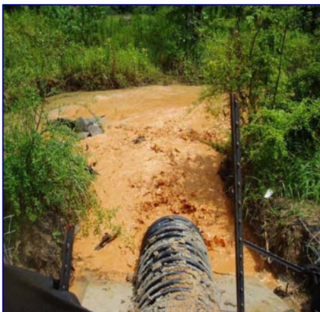
Sediment laden stormwater
