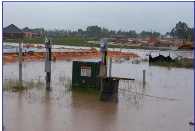
Flooding at development site
