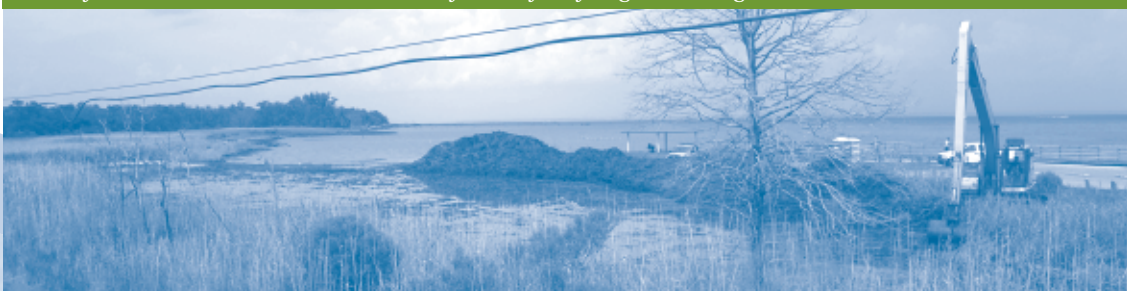
View of the Helen Wood Park marsh excavation from the foot of Dog River Bridge.
