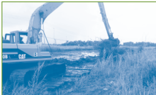
Mitch Dickens of Esfeller Construction operates the long stick excavator at Helen Wood Park
