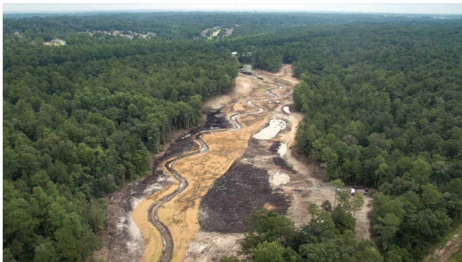
The restoration of D'Olive Creek between I-10 and Highway 90 in Daphne is the largest coastal stream restoration project undertaken in the State. Photo: Ben Bremner
