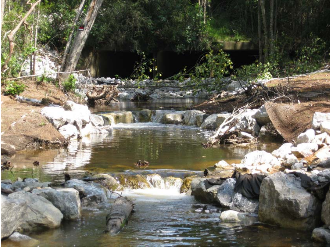
Figure 6.—D'Olive Creek I-10 project monitoring site, highway culverts, and headward erosion restoration.
