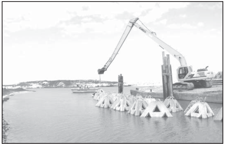
Placement of artificial reef-wave attenuation structures along the shore of Alonzo Landing on the eastern end of Dauphin Island.
