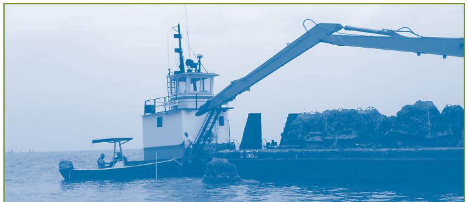
Under the watchful eye of ADCNR and Volkert & Associates, Inc. staff, J&W Marine Construction places the first set of experimental WADS at the Little Bay Restoration site.
