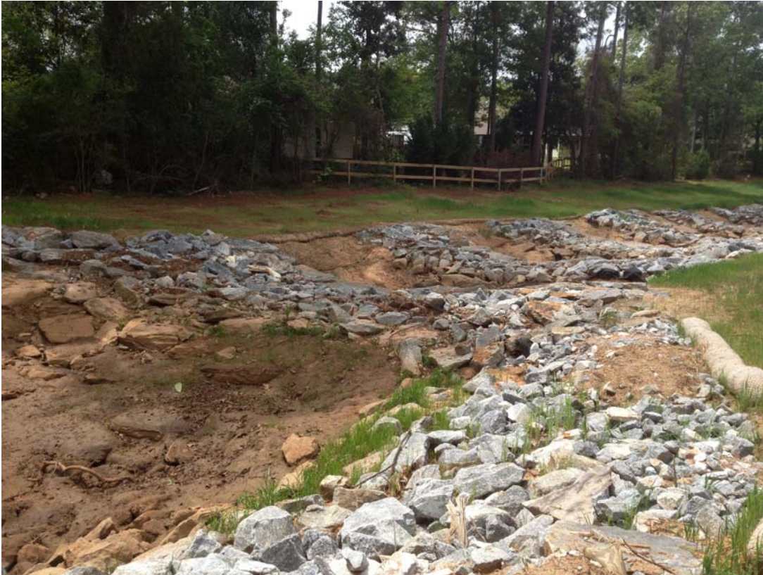
Figure. 1—Step pool conveyance system constructed in the unnamed tributary of Joes Branch in Spanish Fort.
