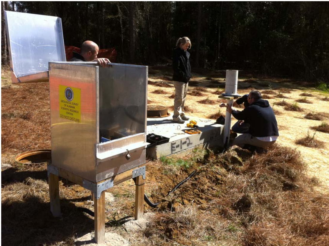
Figure 3.—Installation of discharge and precipitation monitoring and sample collection equipment at Joes Branch site JB1.
