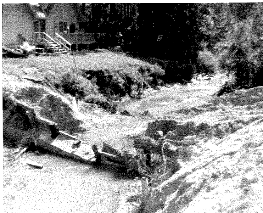
Fig. 10.--Collapsed earthen dam on Tiawasee Creek (John Carlton photo, 1979).
