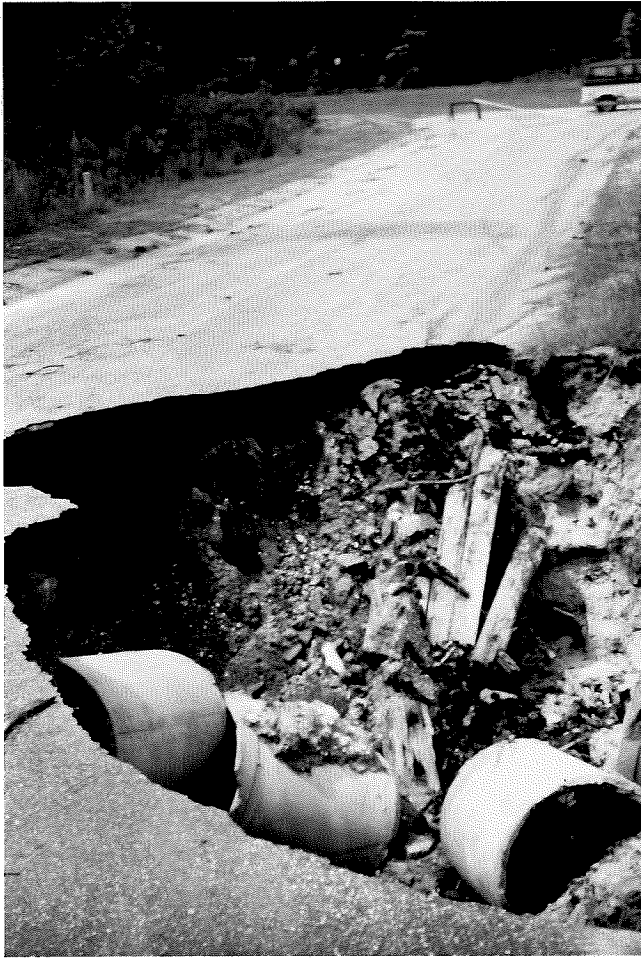
Fig. 16.--Collapsed street in Lake Forest Estates caused by culvert failure and headward erosion of gully (Lake Forest Estates, 1980).
