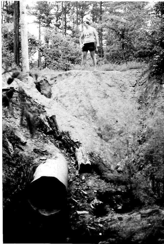
Fig. 19.--Slope failure and exposure of 3 foot diameter, corrugated culvert pipe (Lake Forest Estates, 1980).
