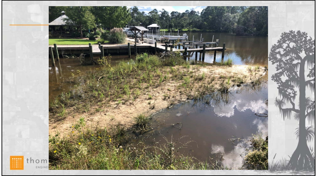
Outfall deposits into Fish River.
