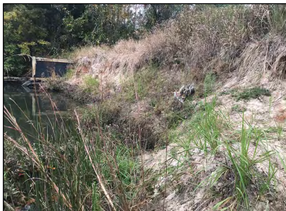
Figure 3.3 Poor quality bank condition at RSA4 (MB 4)
